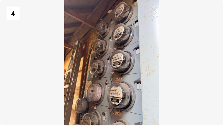
Project: Electrical Room Date: Sep 16, 2025, 1:51 PM Creator: Adam Clements
